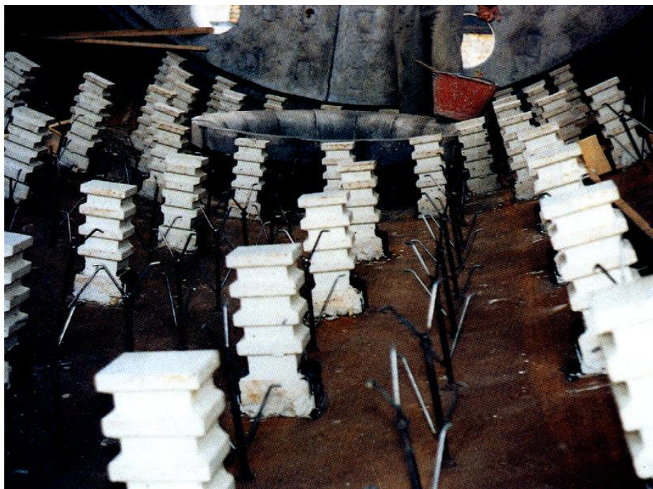
CO Boiler refractory and stainless steel anchoring
